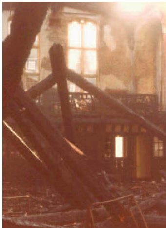
The charred ruins of the interior in the renovation and remodelling of Big School into the College Theatre, which opened on 14 July 1984.
