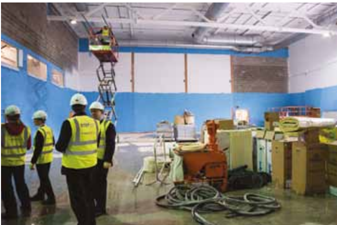
The size and scale of the new sports hall can be seen in this view
