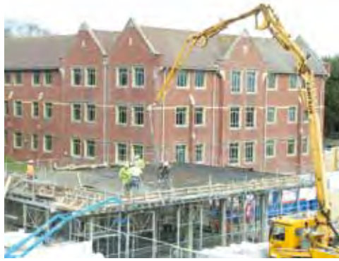
March 2016: Concrete being poured to form the first floor of part of the academic block, in front of the science centre
