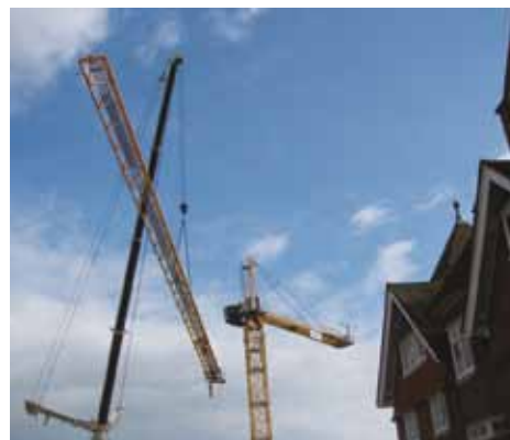
February 2016: A massive mobile crane on the left helps put together the fixed yellow crane on the right, dwarfing the Headmaster's House
