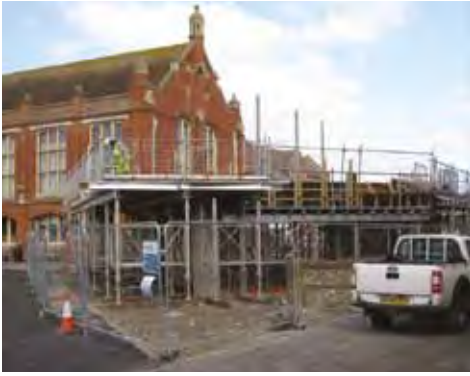
March 2016: The ground floor of the new pavilion begins to take shape
