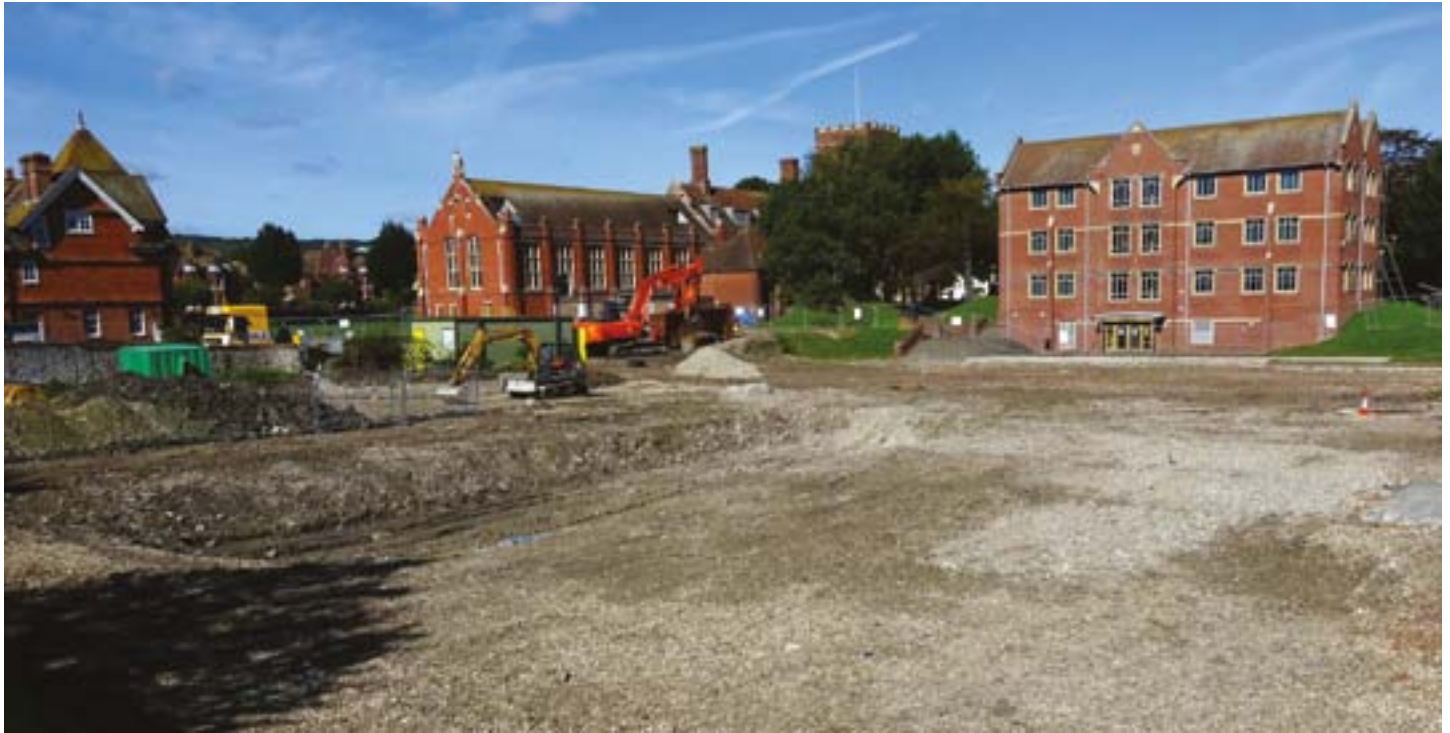
The demolition has opened up new views of the College. This one looks across the Project 150 site from Carlisle Road and shows the Headmaster's House on the left, Big School in the middle and the Science Centre on the right
