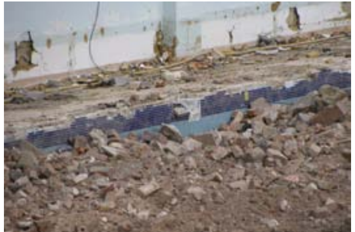
In 2015, with the pool full of rubble, only the tiles remain visible
